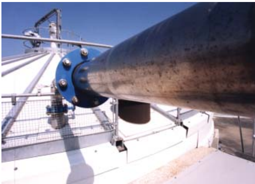
Treatment tanks can be covered and the foul air extracted
