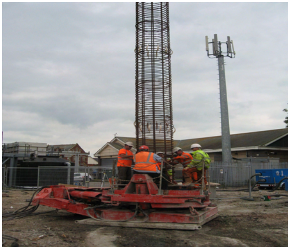
A steel reinforcement cage used during the installation of the pumping station shaft
