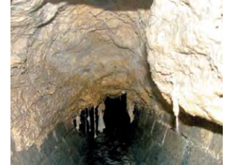
A sewer pipe blocked with FOG
