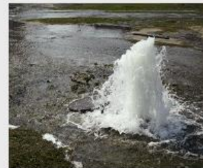
A burst, water is spraying out of the ground
