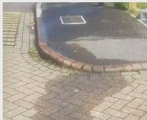
Trickling or a damp patch on the ground
